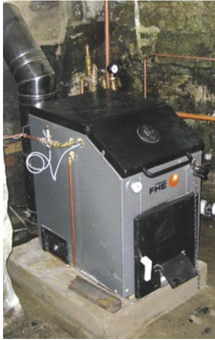
The 60 kW log burning boiler above and 14 kW Kakkelovn below
