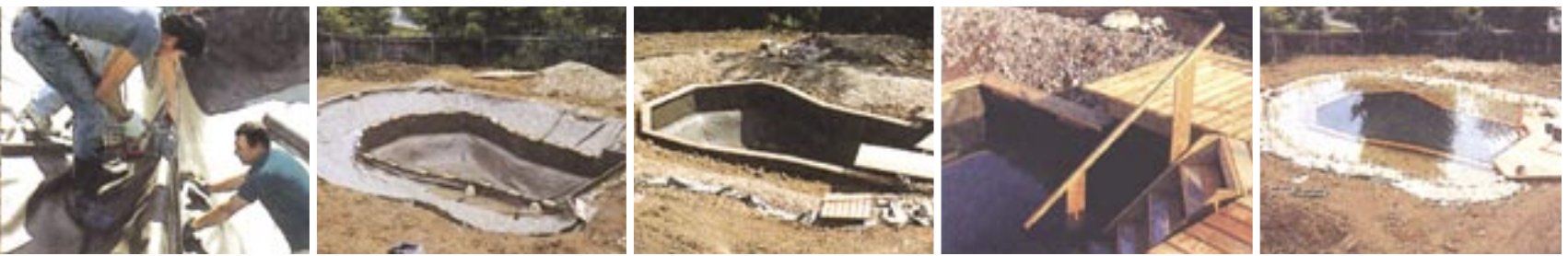
The construction sequence is similar to that of an elaborate garden pond. The important notes to remember are that the swim area walls are kept 100mm below the surface water height to allow water to mix between the swim zone and the plant zones.
